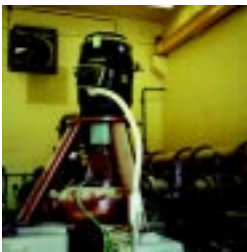
Return Sludge System 75 HP pump
