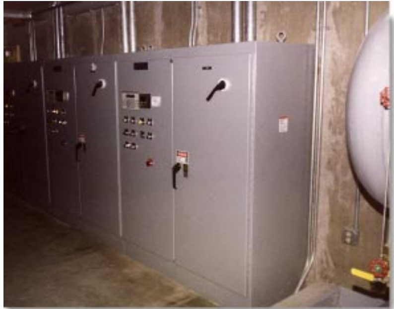
Pump-PAK ™ controllers installed at the City of Grand Rapids Water Department
