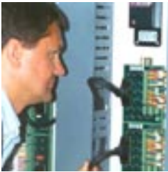
Jim Van De Wege, Superintendent, Holland Water Treatment Plant, inspects Modicon CableFast pre-engineered cable-and-terminal block assemblies. The assemblies, which replace independently wired marshalling blocks and I/O connectors, reduced Windemuller Electric's cabinet fabrication and test labor by 200 manhours over five cabinets
