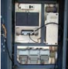
Panel close up showing Momentum PLC, radio, batteries and power supplies.
