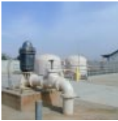
Wellsite with treatment vessels in background.
