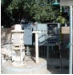
Well with PLC panel (R).
