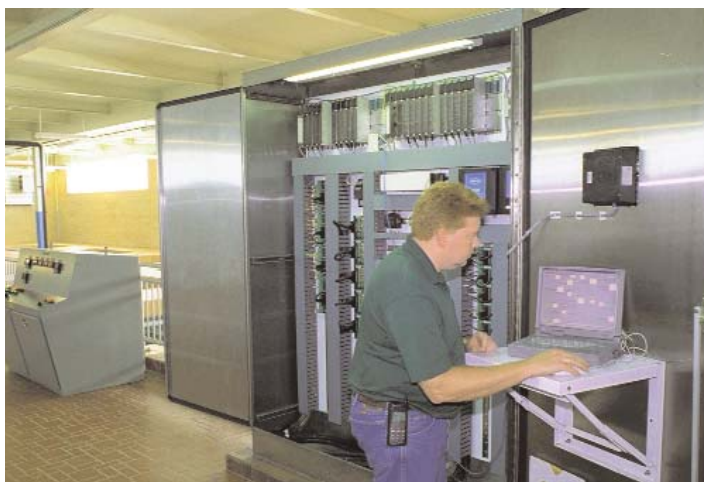
INSTRUMENT CONFIGURATION CAN HAVE A DRAMATIC EFFECT ON A PLC-BASED CONTROL SYSTEM. FOR EXAMPLE, A MISCONFIGURED TURBIDIMETER INTERFACE COULD CAUSE A PERMIT COMPLIANCE ISSUE OR INEFFICIENT OPERATION.
